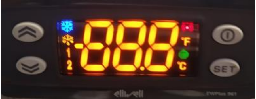
Fig. 3.3.1. Indication and control elements of the controller Eliwell.
